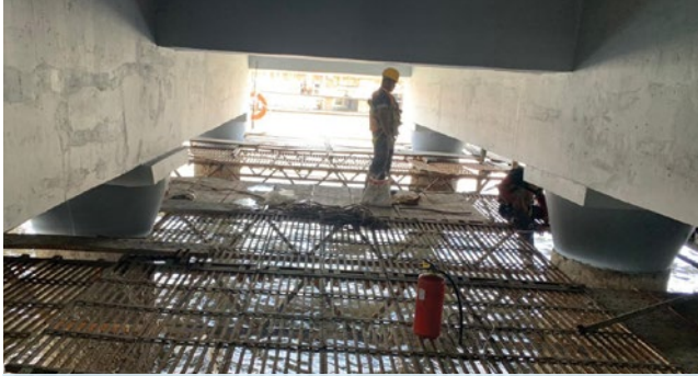
Restoration of RCC Elements Corrosion treatment, concrete section built up & protective coating
