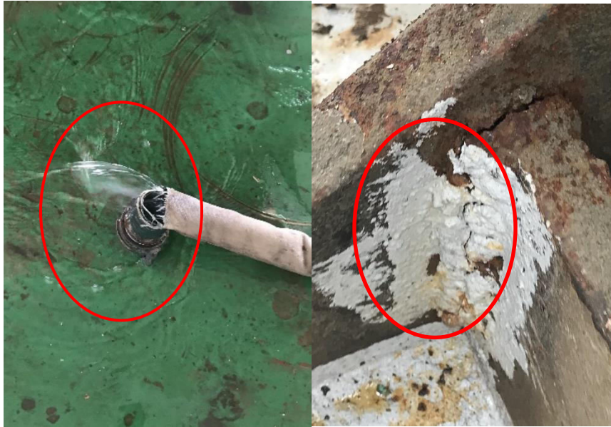
Figures 2 and 3: Burst fire hose (left) and cracked weld (right).
